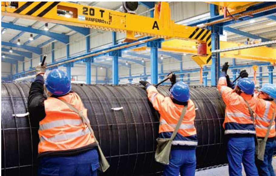
Workers installing equipment for the Nord Stream gas pipeline that will link Russia and the European Union via the Baltic Sea.
